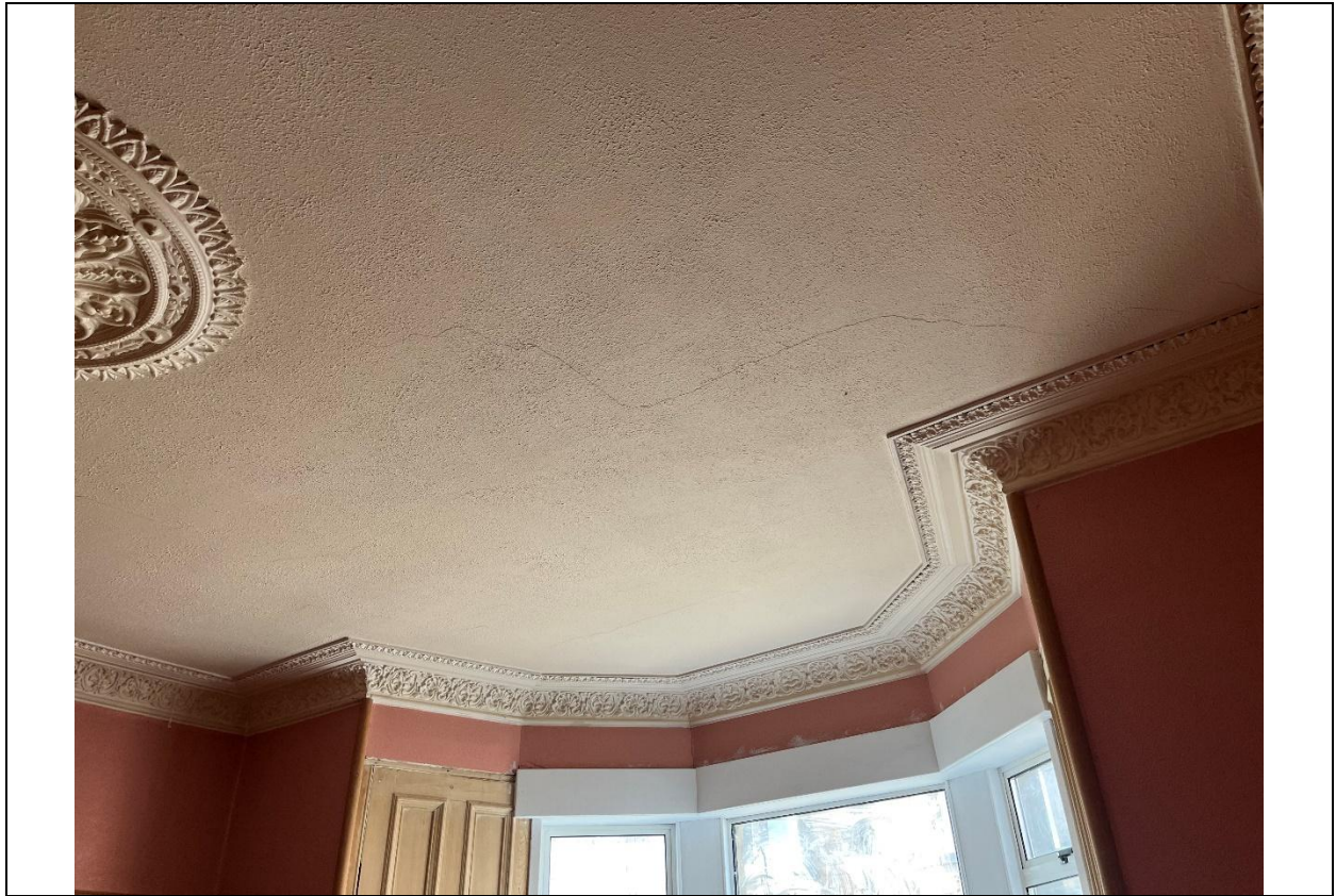
Figure 5 – Typical non-structural cracking to ceilings.
