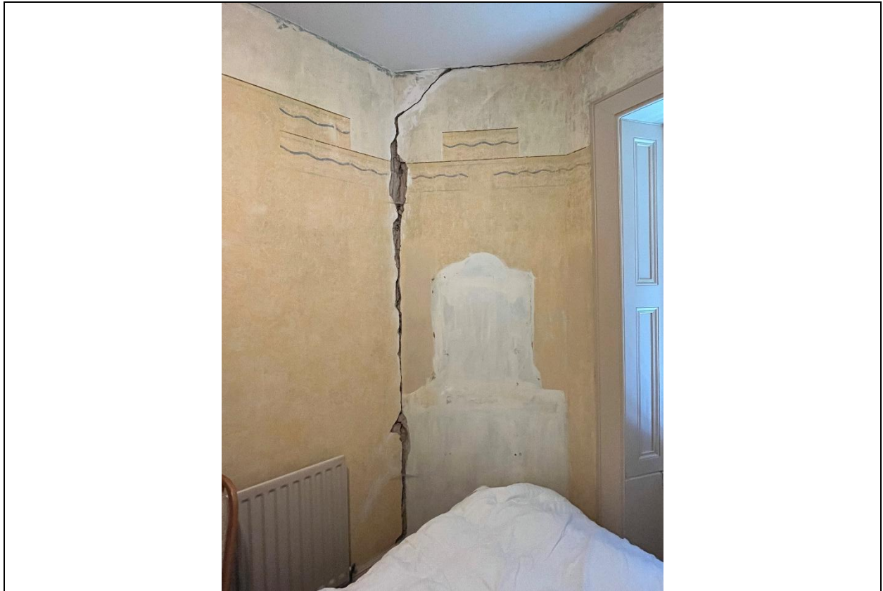
Figure 1 – Pronounced vertical crack to bedroom external/party wall.
