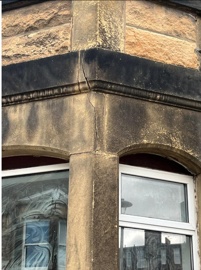
Figure 8 – Cracking to bay-window lintel bearing.
